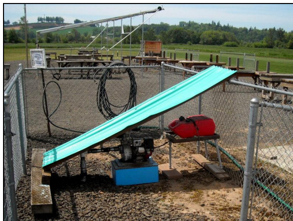
Pump back on the well.
